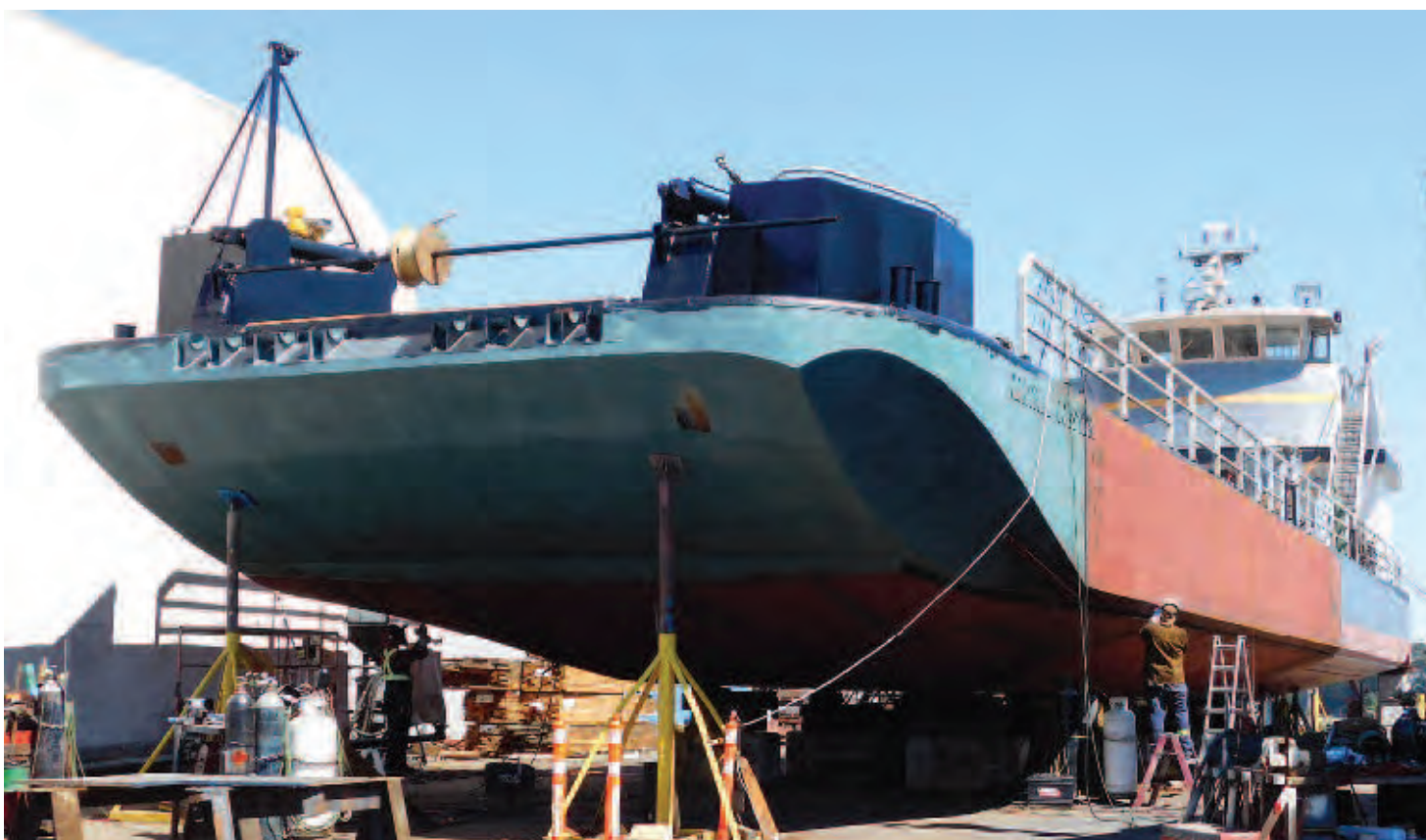
LEFT The Central Coaster's new 60-foot double-hulled midsection was fabricated by Canron Western Constructors in Delta, and welded in place between the refitted original bow and the new 30-ft extension at the stern.
