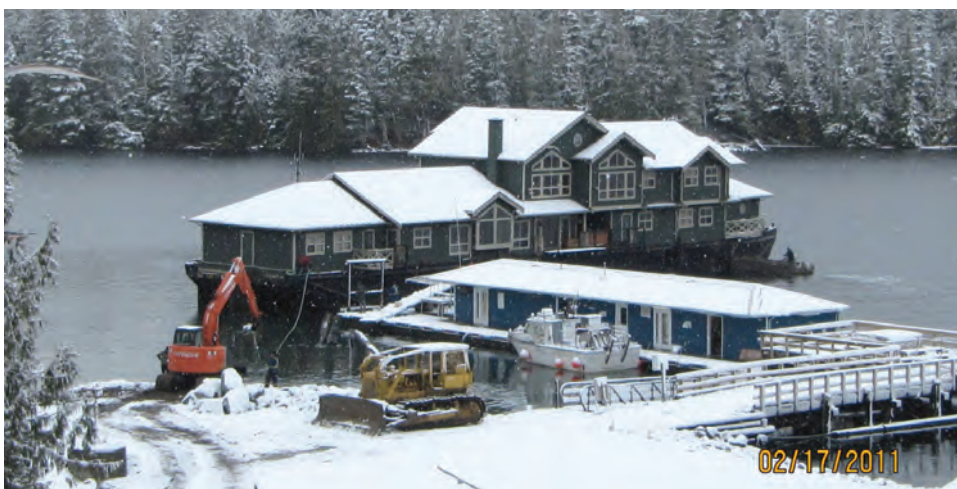
The "Big Time Sportfishing Resort" declared bankruptcy and assets were auctioned off in Nanaimo. Craig purchased the fully outfitted 20-room lodge for $225,000 and moved it to Shearwater.
