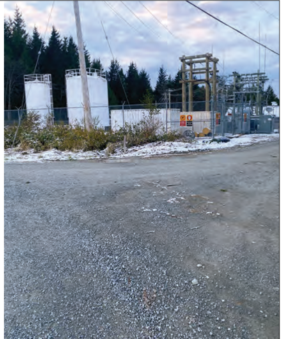
BC Hydro's Transmission Yard and Fuel Depot near Shearwater on Denny Island.
